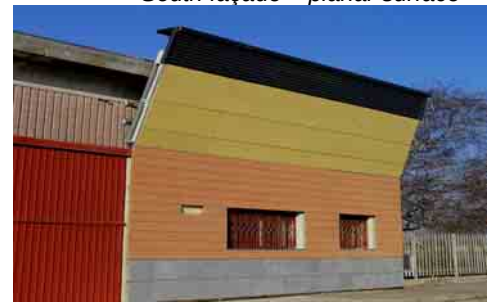
East façade – partially tilted
